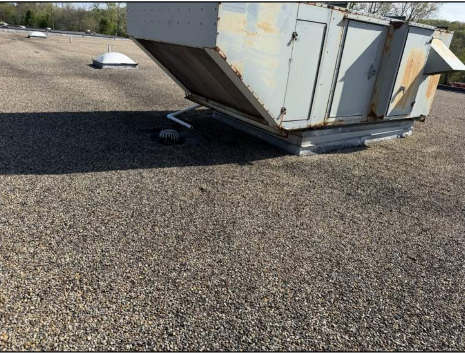
EXISTING ROOF TOP UNIT
