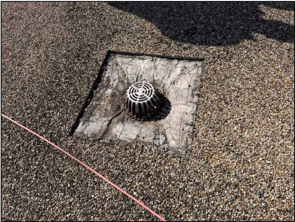
ROOF DRAIN PICTURE
